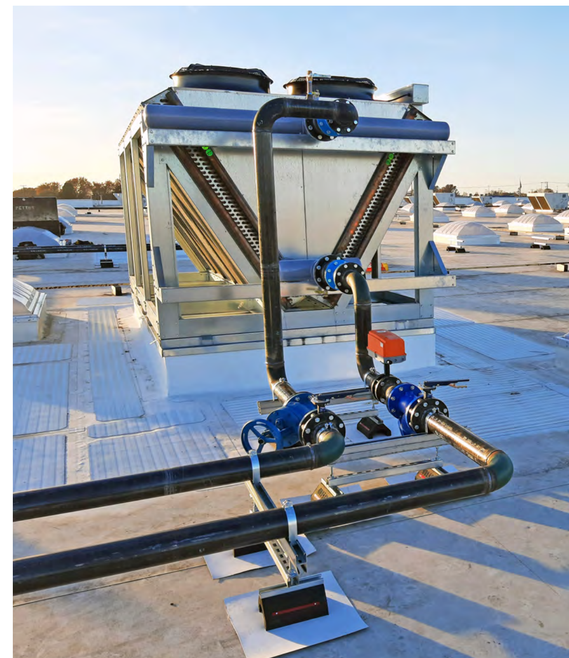
Dry cooler used to reject heat from a water-source heat pump using glycol as the fluid
