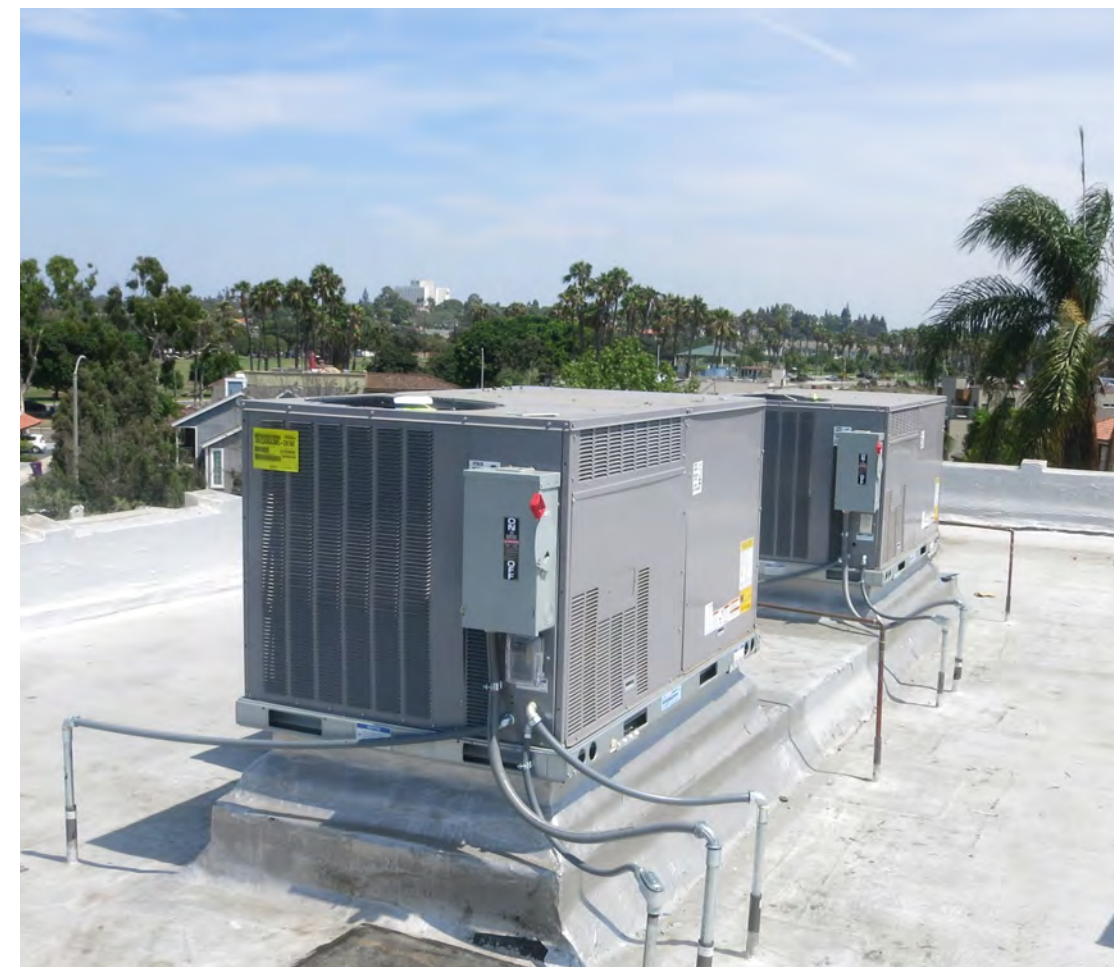
5 ton rooftop heat pump.
