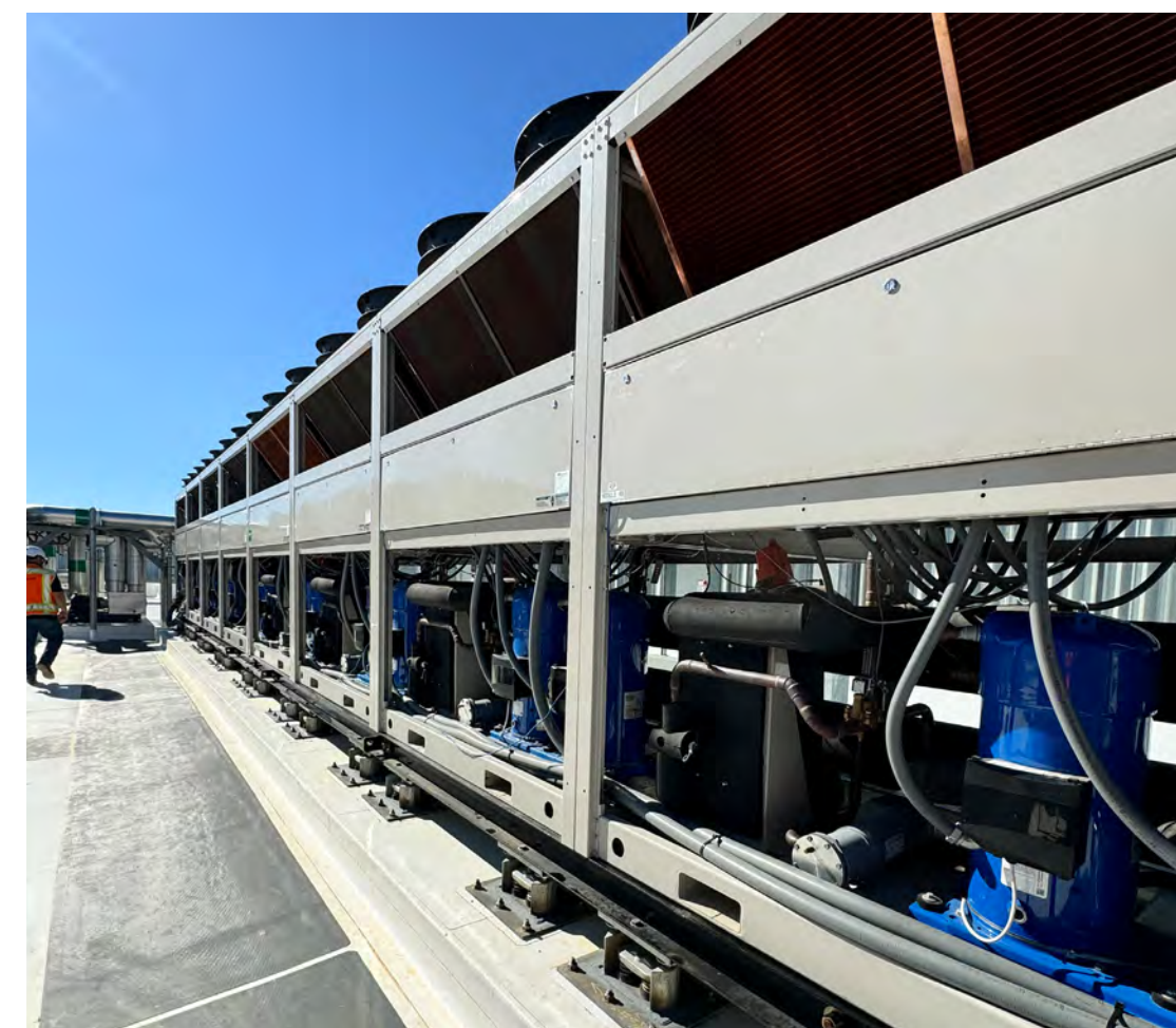
Multiple 4-pipe air-to-water heat pumps stacked together for 480 tons of cooling and 240 tons of heating.
